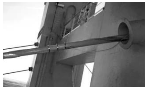
c) Wire breakage of bridge multi-layer strand cable
