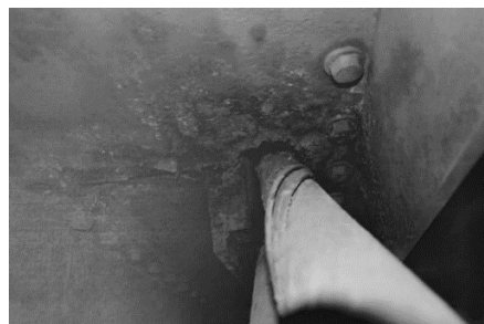
b) Wire breakage of bridge multi-layer strand cable
