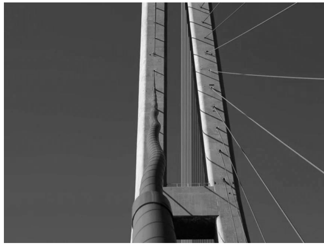
a) Stay cable pipe "waviness"
