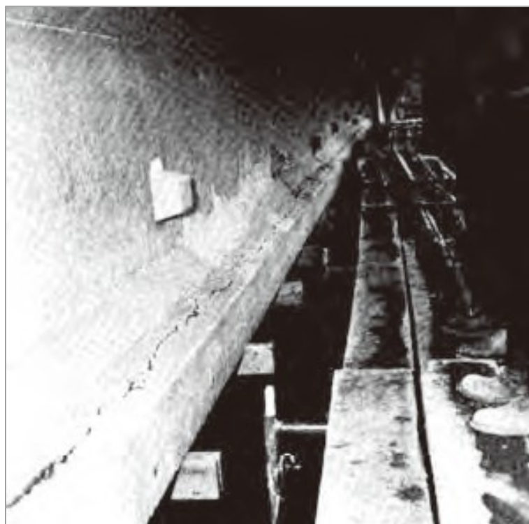
Figure 15 Longitudinal crack on the outer sloping face of the bottom flange (south facia girder)
