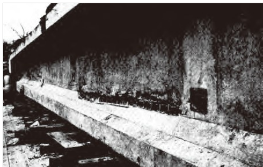
Figure 14 Honeycombs in the first girder cast in 1949
