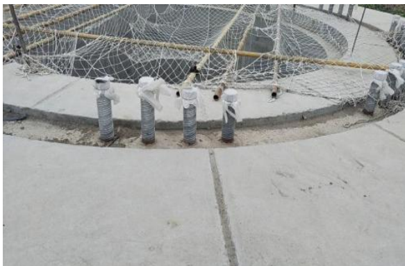
Figure 2 Grooves in the interface between the foundation and concrete tower
