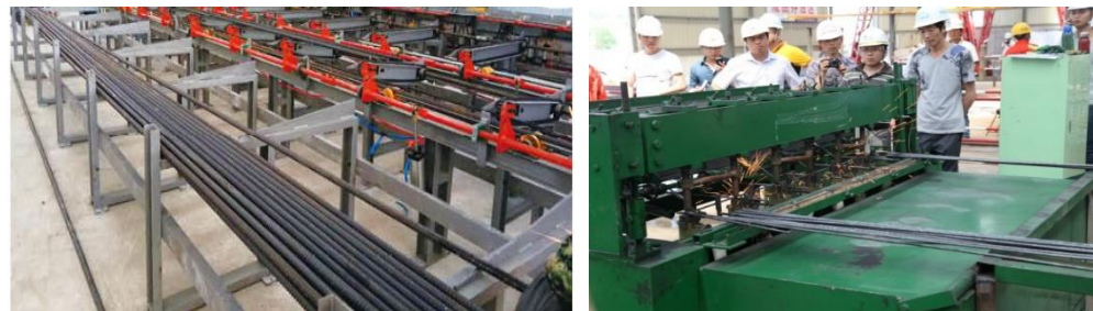
a) CNC steel bar sawing and cutting b) Fully automatic mat reinforcement welding
