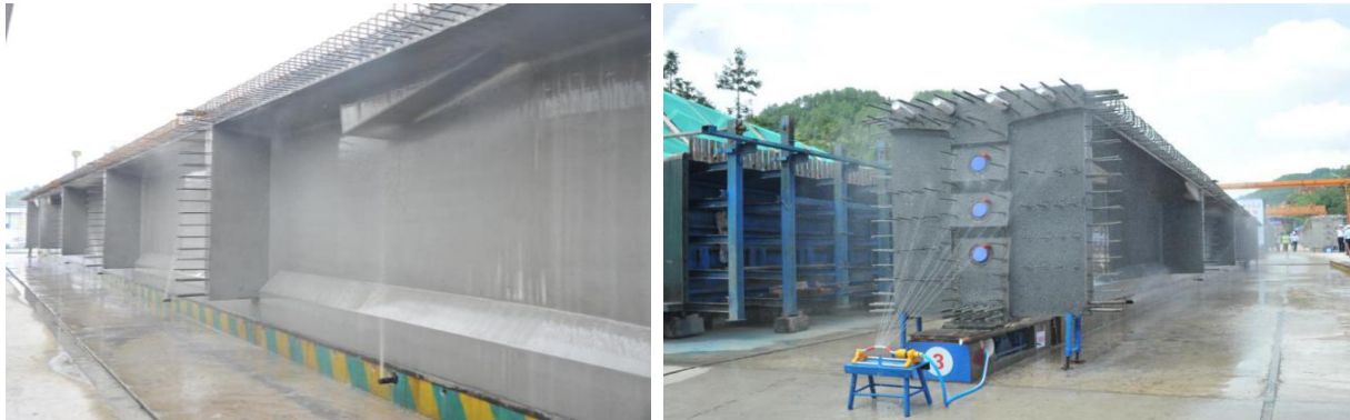
Figure 9 Intelligent curing system
