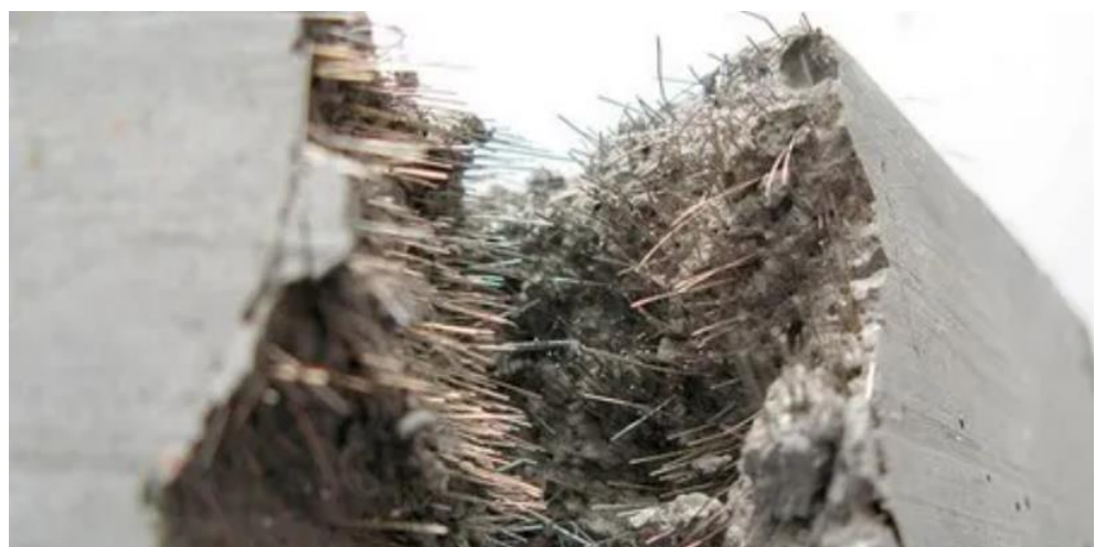
Figure 2 UHPC structural failure surface
