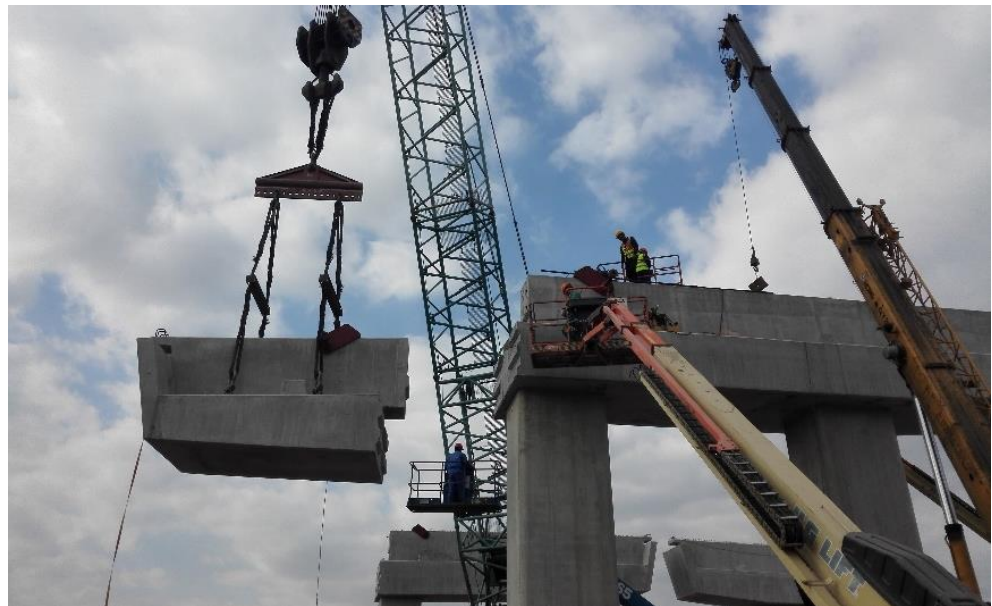
Figure 10 Construction of a three-section bracket joint bent cap of S7 in Shanghai
