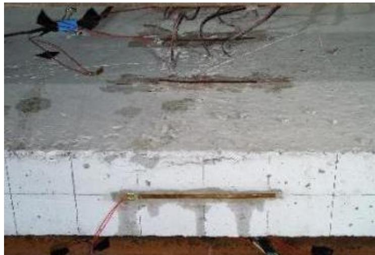
Figure 5. Surface cracks on concrete slab of second beam
