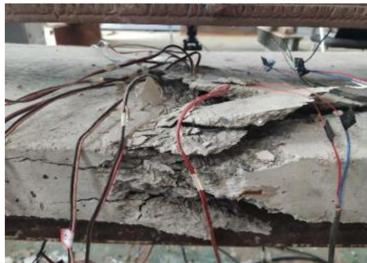
Figure 4. The crush state of the concrete of the reference beam
